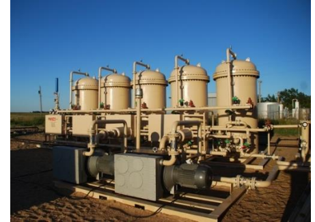
Modular units used to treat the raw gas stream to remove nitrogen, CO2 and concentrate helium
